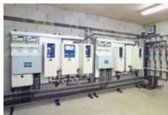
Duty/Standby Chlorine Gas Feeder Systems
