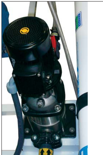
Raw Seawater SS Feed Pump
