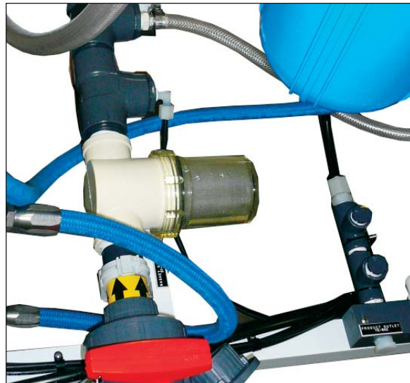
Inlet Seawater Strainer
