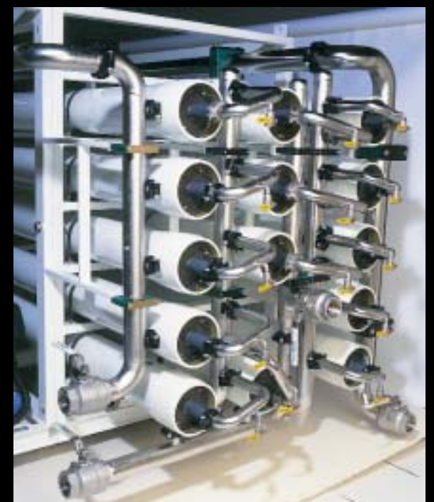
Stainless Steel HP Piping
