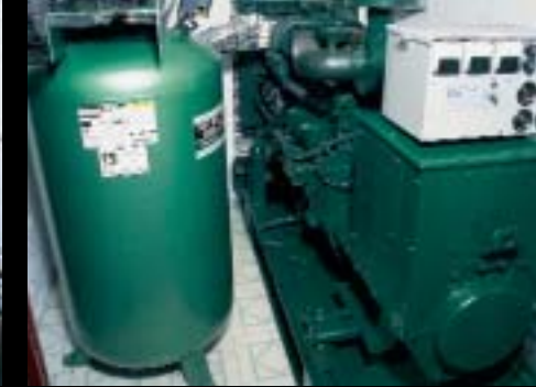
Optional Installed Generator, Air Compressor & A.C.
