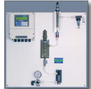
Series 4000 Transmitter, CL4000 and pH Probes on Flow Control Panel
