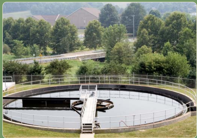
Constructed in 1980, the Lititz Sewer Authority Wastewater Treatment Plant has undergone numerous retrofits and modifications.
