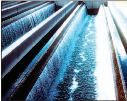
Village Creek stormwater filters in operation. The facility's 22 filters are laid out in two trains with room for expansion.
